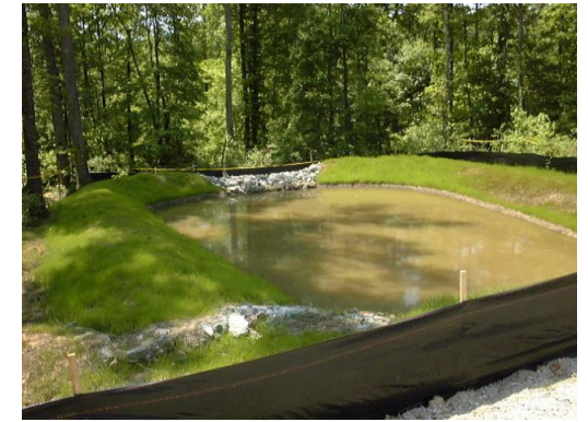
An example of sediment trap and silt fence. Note the vegetative stabilization on sediment trap berm.
